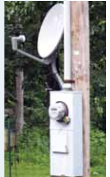
Satellite dishes and other unauthorized attachments must be removed to protect lineworkers.
