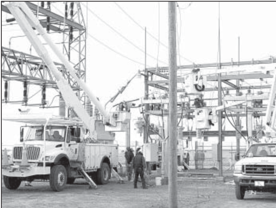
Lane-Scott's crews and High Line Services crews working on the Manning Substation.
